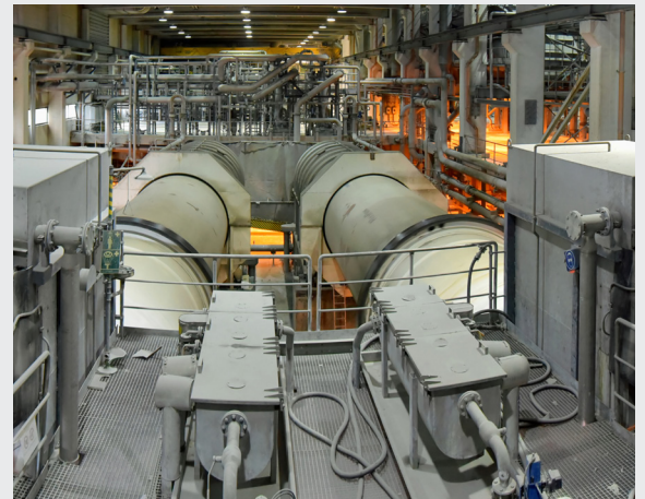
Compressed air systems are a critical component of the paper recycling process
