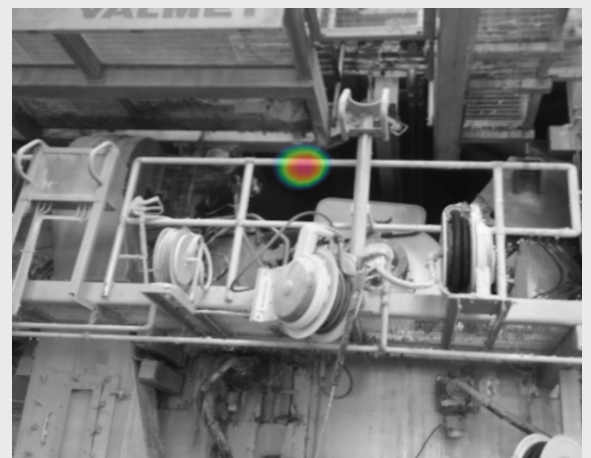
The FLIR Si124 detecting a compressed air leak
